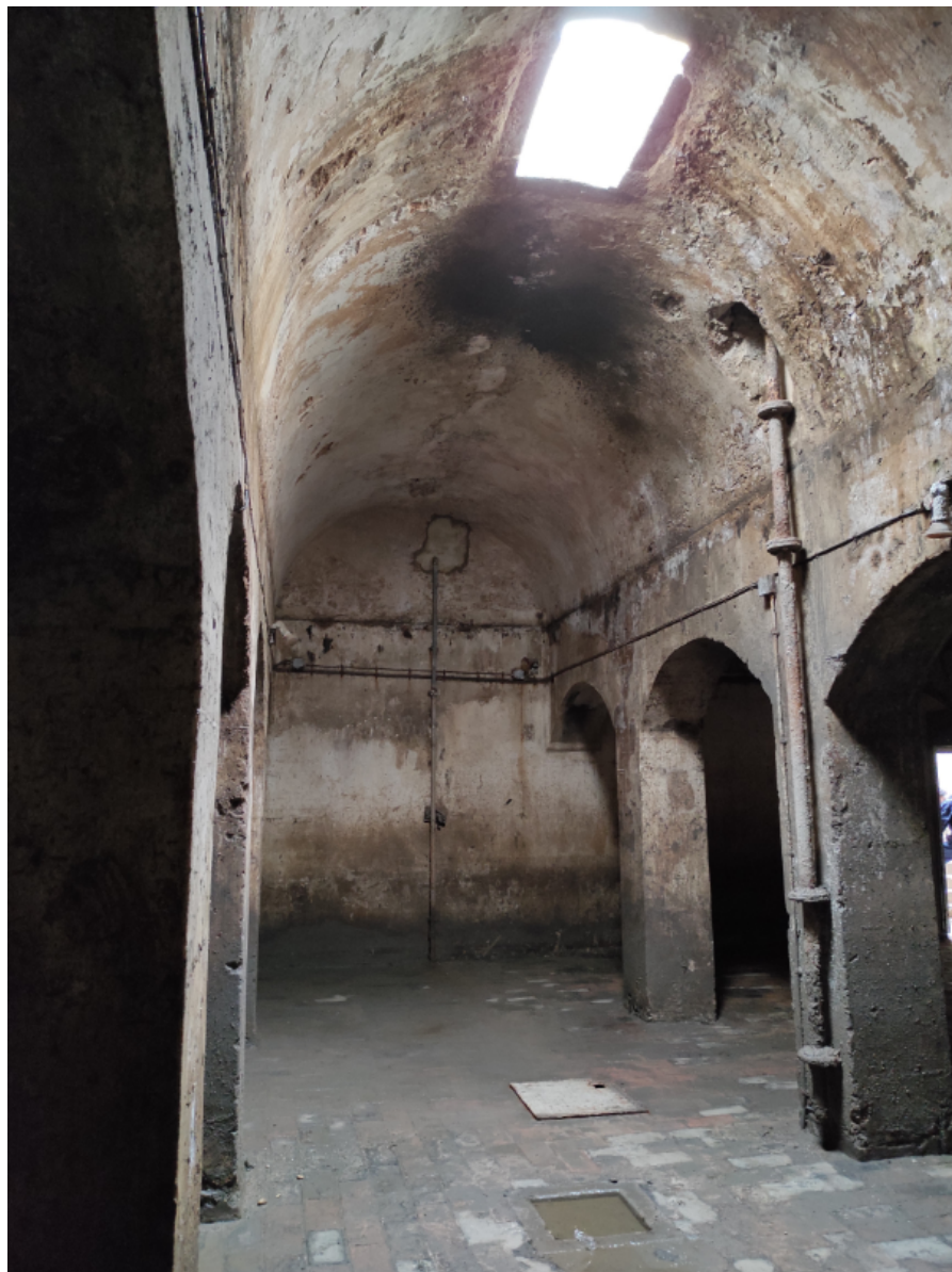
Nun's Well, Europa Flats, now open to the public. An underground reservoir thought to date to the medieval, Moorish period, though it may be earlier; it is the earliest structure linked to water supply in Gibraltar. Its interior is whitewashed with lime.
