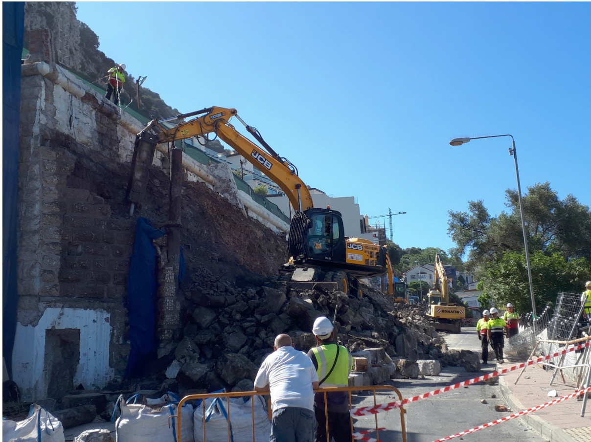
Demolition of the late 19 th -century blast wall erected originally to protect the two huge historic water tanks on Europa Road in August 2021. The demolition was monitored by archaeologists from the Gibraltar National Museum, funded by the developer. The tanks themselves are to be preserved within The Reserve residential development and the demolition revealed the original limestone façade. The development will also re-use material from the catch pits in an iconic entrance and include information on the site's history for residents and visitors.
